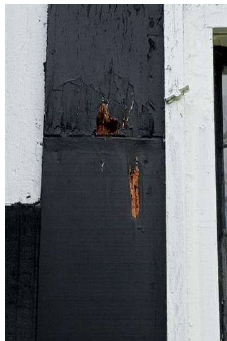
There are two small rot pockets in the timbers next to the window, nearest the addition
