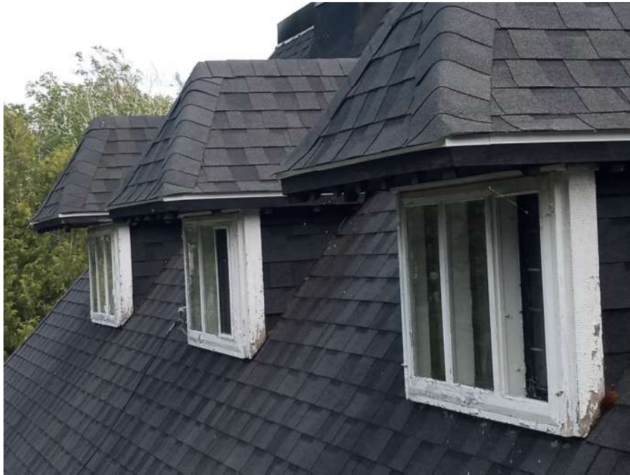
The four dormer windows on the back elevation, 3B1, 3B2, 3B3 and 3B4, have peeling paint on the exterior side trim. The storms are typical of 2F3-S.
