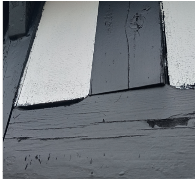
In this one, there is plywood over the original panel
